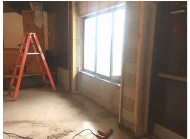
The old walls are removed and the space is prepared for new walls.
